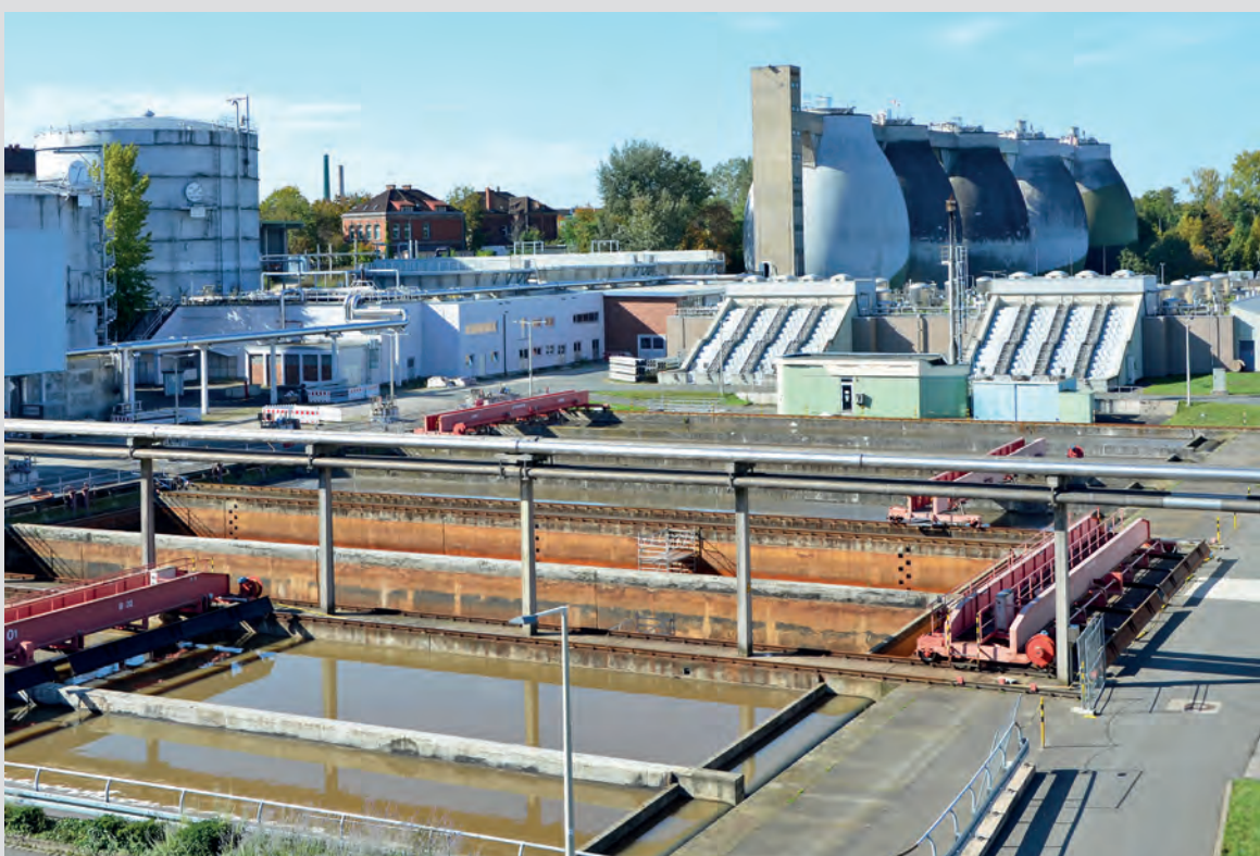
Sewage Treatment Plant No. : Sedimentation tanks, first biological stage, sludge digester. Photo: Susanne Vogel (SUN).
