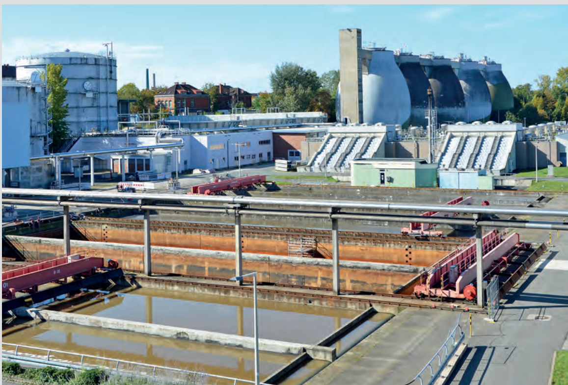
Sewage Treatment Plant No. 1: Sedimentation tanks, first biological stage, sludge digester. Photo: Susanne Vogel (SUN).
